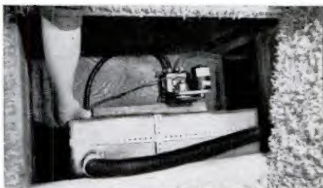
WATER PUMP , easily accessible, is neatly hidden from view under cutaway section of carpeted deck
